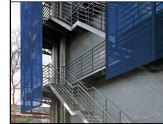
ADAPTING EXISTING TECHNOLOGIES REFERENCING A BUILDING UNDER CONSTRUCTION, A LAYER OF BLUE METAL MESH, WRAPS AROUND THE ENTIRE BUILDING SUPPORTED BY A SCAFFOLD
